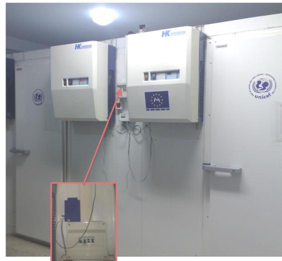
Figure 5: FoneAstra deployed at IPH in Tirana, Albania. The FoneAstra box is placed between the two compressors for two cold rooms (note door handles on left and right). Wires from the board pass through thermally insulated holes in the walls of the cold rooms and lead to the sensors inside.
